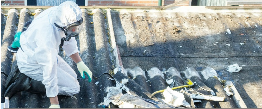
Asbestos abatement focuses on either removing it or enclosing it so fibres cannot be released. The hazard presented can vary from high to relatively low depending on the concentration of dust in the atmosphere and the availability of ventilation or extraction (though it is worth noting that The Mesothelioma Centre states "any amount of asbestos exposure can cause serious health defects.")
